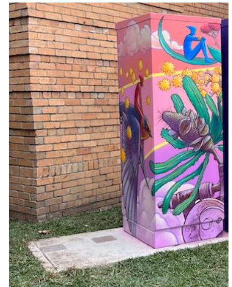
Figure 10: The concrete pad was installed with space for an additional panel in the future.
